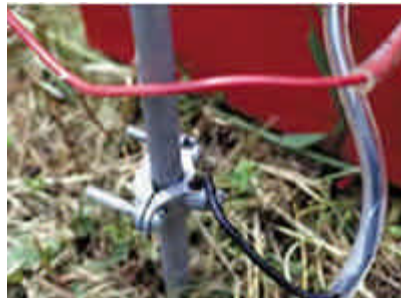
7. Metal ground rod.
